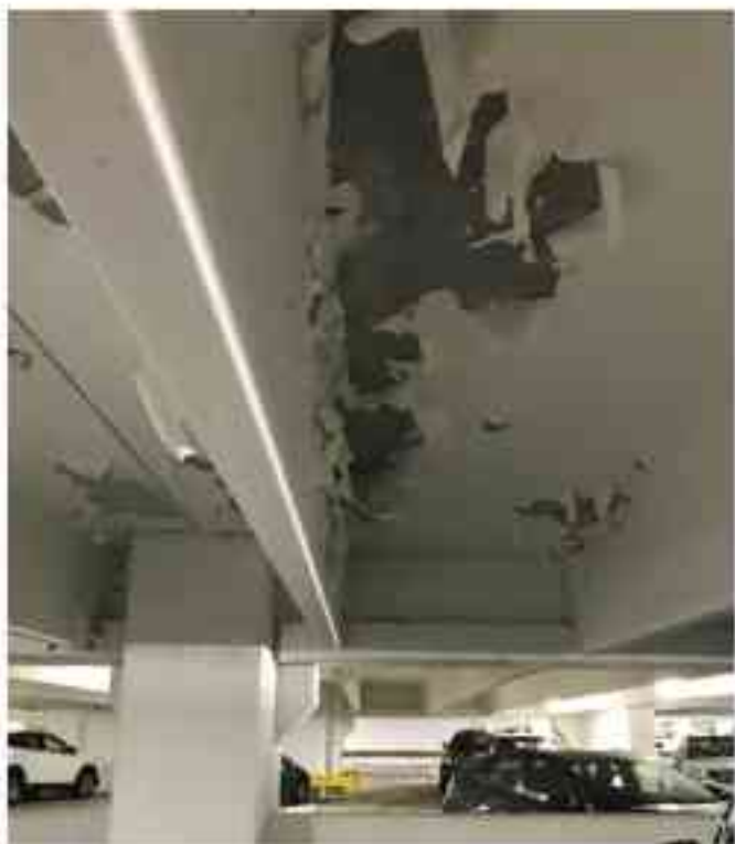
Fig. 5: The coating failures were widespread in many areas
