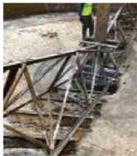
Fig. 1: Damaged gravity thickener rake arm mechanism. PHOTO COURTESY OF THE AUTHOR UNLESS OTHERWISE NOTED
