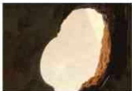
Fig. 4: Galvanic corrosion at bolted connection
