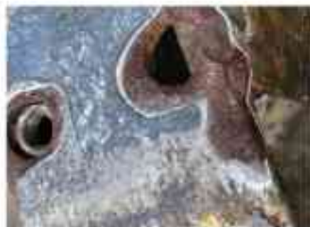
Fig. 14: Clear evidence of galvanic corrosion of the carbon steel at bolt holes where the stainless steel fasteners connected the scraper blades to the rake arms. These were round bolt holes before edge corrosion losses widened the holes.
