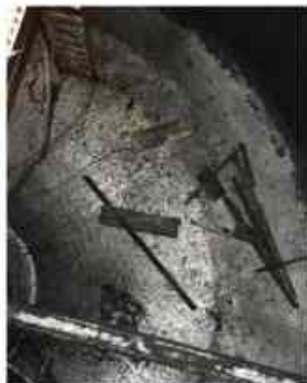
Fig. 2: Damage to clarifier bottom
