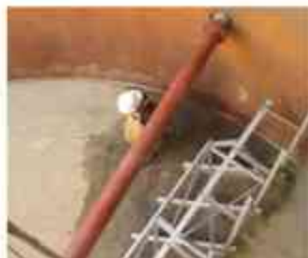
Fig. 7: Rake arms in 2015, prior to entering into service
