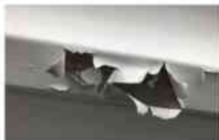
Fig. 3: Spots of tightly adhered coating within the area of delamination
