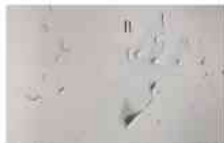
Fig. 4: The coating was partially removed during the cleaning and painting process. The edges of the intact coating lifted as a result.
