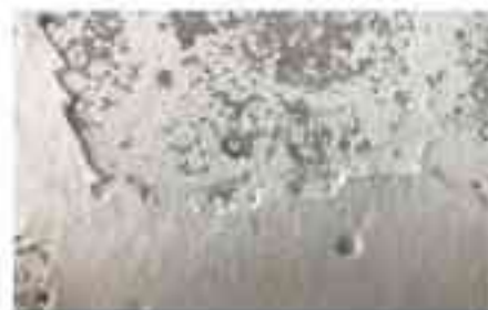
Fig. 2: Close-up of weak, crumbly coating left on surface after the newly applied coating delaminated
