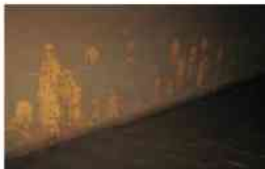
Fig. 1: Evidence of reinforcing steel corrosion on the lower wall of a concrete channel FIGURES COURTESY OF THE AUTHOR (UNLESS OTHERWISE NOTED)
