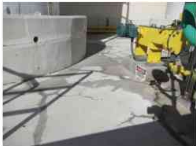
Fig. 6: Severe cracking on the floor of a secondary containment structure
