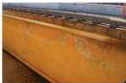
Fig. 8: Existing 30-year-old coating with delaminations had to be evaluated
