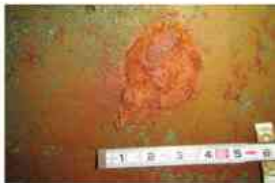
Fig. 2: Detail of corrosion nodule forming on the surface of a concrete wall
