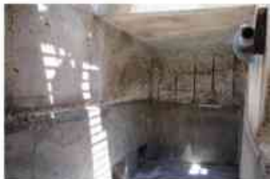
Fig. 3: Biogenic corrosion of concrete above the wastewater surface
