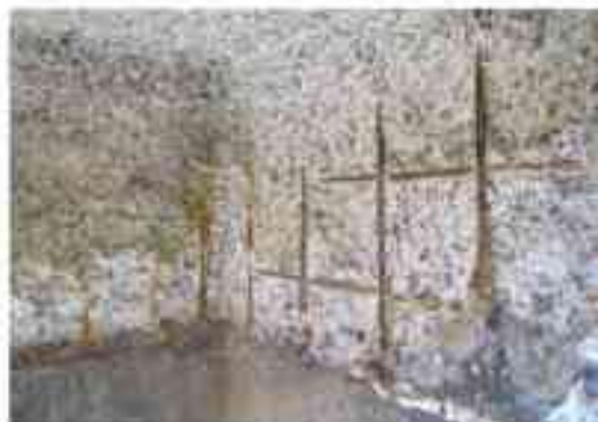
Fig. 4: Deterioration of concrete has exposed and completely corroded the reinforcing steel
