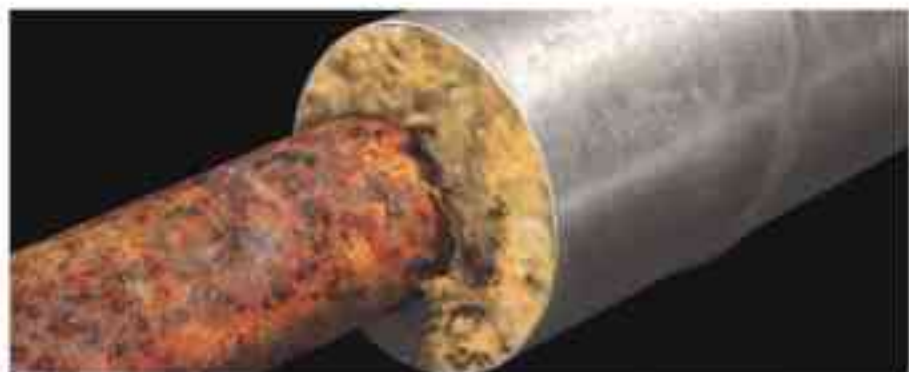
Fig. 1: An example of corrosion under insulation, showing severely deteriorated steel underneath the insulation material.
