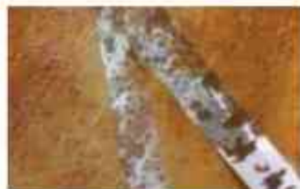
Fig. 8: Adhesion test tape was applied per ASTM D3359, but without scribing. The back of the tape and underlying surface are shown as the tape was being removed.
