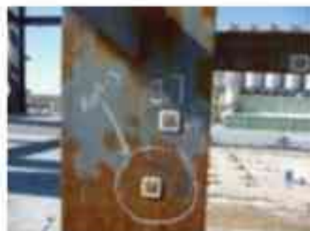
Fig. 5: Visual example of a corrosion zone on one of the supplied columns (Column J-7).
