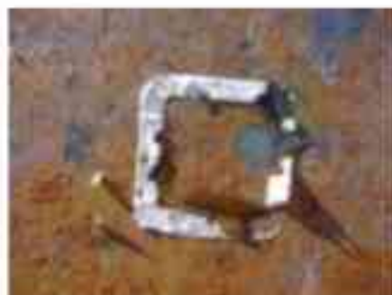
Fig. 6: This example shows a crust-like material, stained coating, blisters and substrate corrosion.
