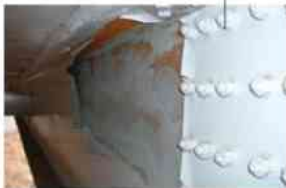
Fig. 1: Failure of incompletely cured inorganic zinc-rich primer. All coats were shop-applied. Photos courtesy of KTA-Tator, Inc.
