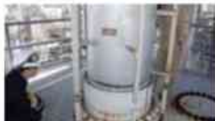
Inspection of TMIC after one year in service showing no coating breakdown or rusting. Photo courtesy of the authors.
