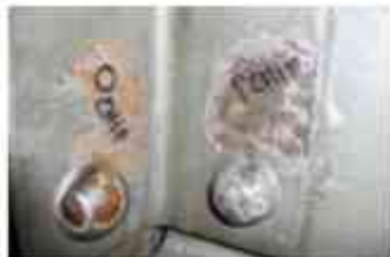
The left side of the angle shows old primer; the right side does not. Photo courtesy of KTA-Tator, Inc.
