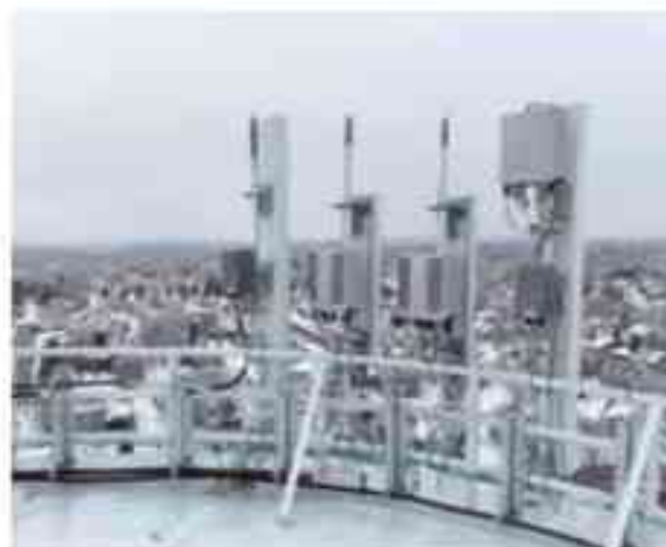
Fig. 1 (facing page): Elevated water storage tanks are commonly used for telecommunications equipment installation. Photos courtesy of the author.
