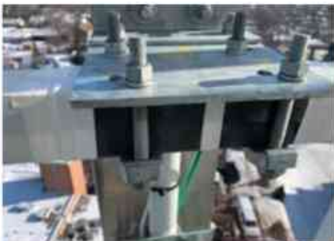
Fig. 5: Galvanized compression plate assembly used for attachment of the antenna support pipe to the handrail system.
