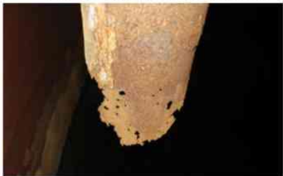
Fig. 2: Left unchecked, coating failure can result in significant metal loss, as seen on this pipe in a tank interior.
