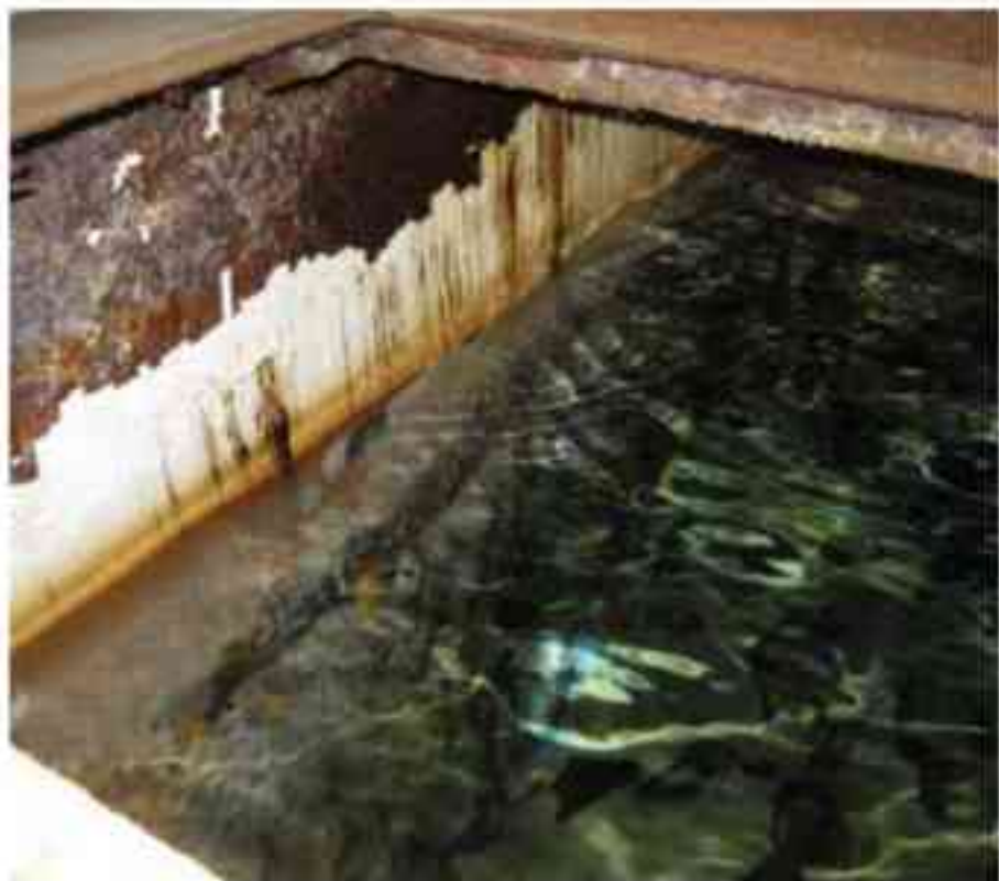
Fig. 2: Severe corrosion above the water line (the ultraviolet) is a common mode of failure. Moisture-vapor molecules are smaller and more insidious than liquid water molecules, and are able to permeate the coating system faster than liquid water, thus leading to accelerated corrosion. Photos courtesy of the author, unless otherwise noted.
