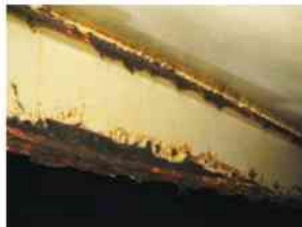
Fig. 1: Corrosion and metal loss on a roof rafter. Photos courtesy of the author unless otherwise noted.
