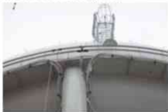
Fig. 3: Use of manufactured colored cabling.
