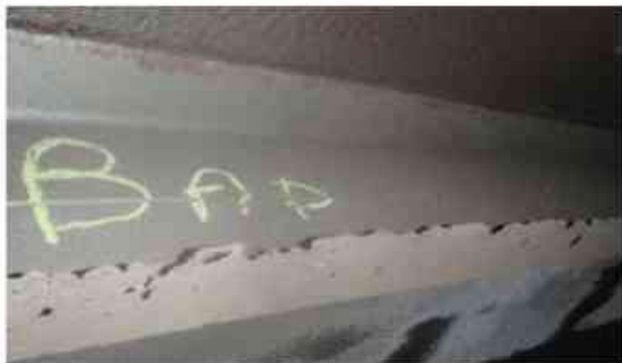
Fig. 3: A roof rafter with metal loss exposed following interior cleaning.
