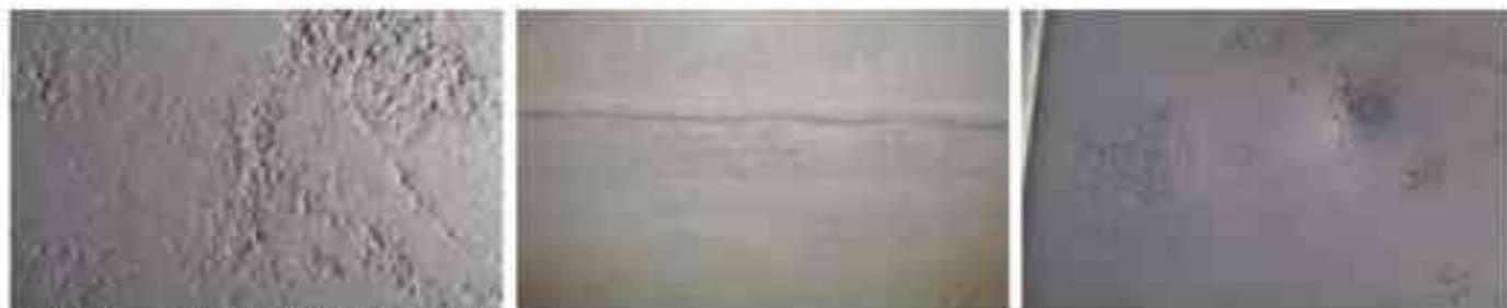
Fig. 4: Pitting as evidenced in corroded steel tank bottoms.
