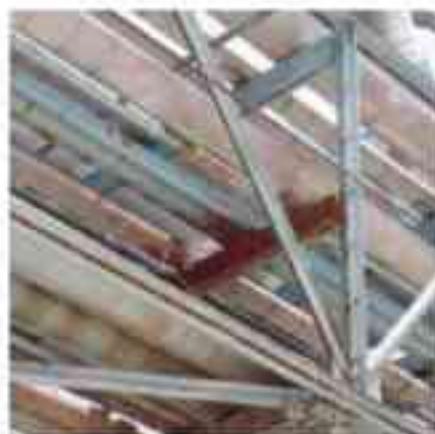
Fig. 3: An overhead rack stuffed with pipes, many of them insulated, is ideal for a thermal-imaging-camera survey, which can be done from ground level and will quickly show which pipes have problems with insulation, jacketing and possibly CUI.
