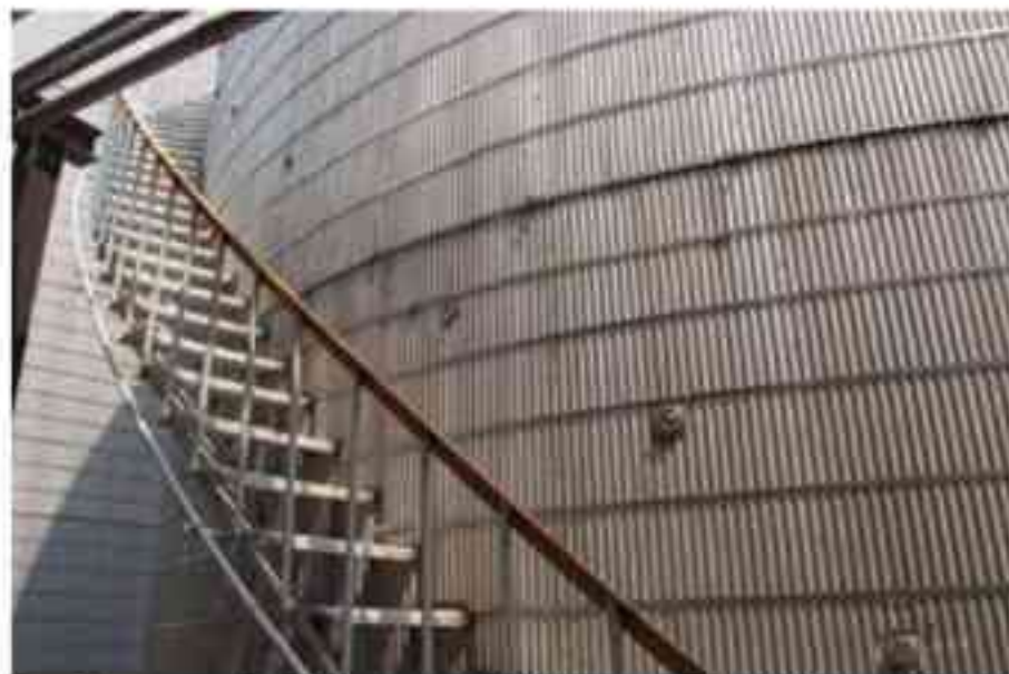
Fig. 1: Older storage tank with OSHA 1910.119 wall-thickness inspection ports placed for easy access along the stairs. This is not where major corrosion is expected to occur. All figures courtesy of the author unless otherwise noted.
