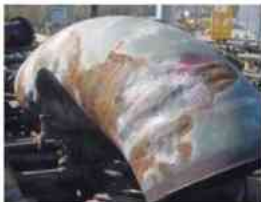
Fig. 1: CUI has eaten away at the surface of this process pipe, which was previously covered with a traditional insulation and cladding system. Figures courtesy of Sherwin-Williams Protective & Marine.
