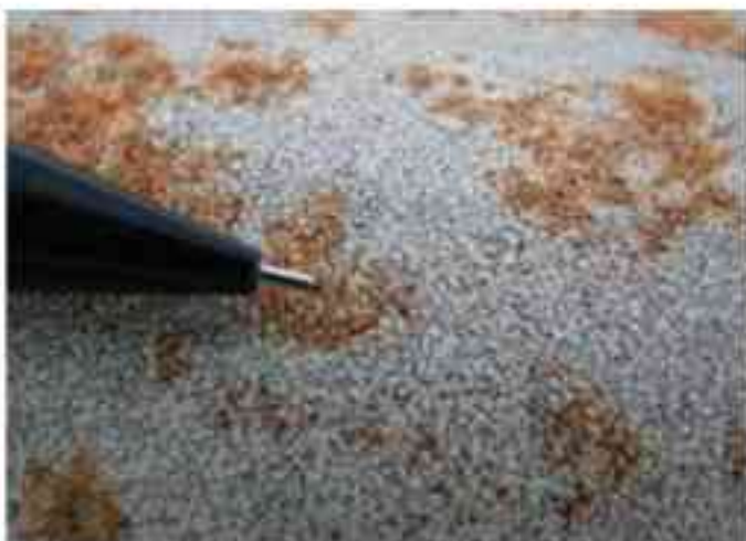
Fig. 5: Close-up of the rough, porous surface.
