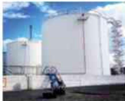
Fig. 3: Processing tanks coated with thermal insulative coatings protect personnel from burns, without the threat of hidden CUI.
