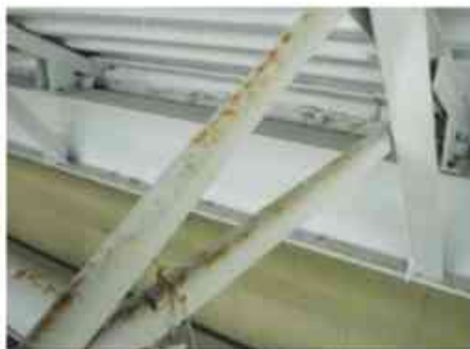
Fig. 2: Rusting on the top surfaces.
