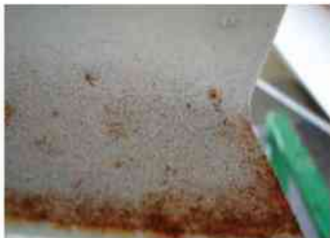
Fig. 4: Representative condition of the coating.
