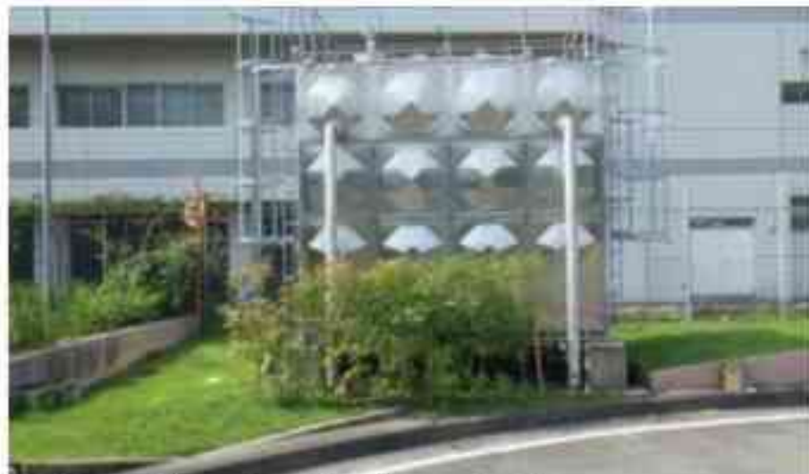
Fig. 2: A stainless steel water-storage tank, one of the unique types of water-storage tanks encountered at naval facilities worldwide.
