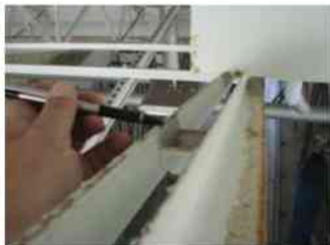
Fig. 3: Close-up of rusting on the top surfaces.
