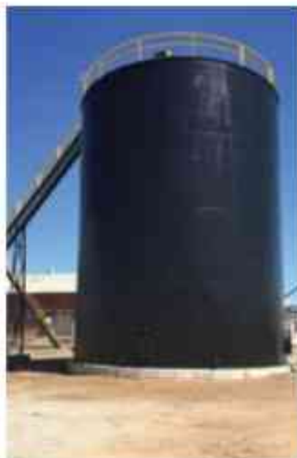
Fig. 5: Although this asphalt tank operates at up to 220 F (104 C), five coats of spray-applied insulative coating provide a safe-to-touch surface, while also helping to conserve process heat.
