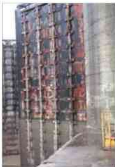
Fig. 6: The exterior of a meter gate showing advanced corrosion.
