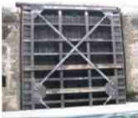
Fig. 4: A single-skinned miter gate with a 60-year-old vinyl-coating system.
