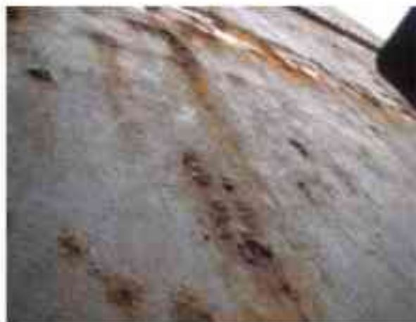
Fig. 3: Some pitting on the old vinyl system that was mostly intact.
