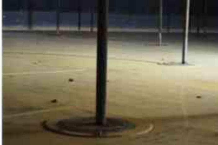
Fig. 2: A leg supporting the floating roof is surrounded by small repairs to the epoxy coating (caused by mechanical damage during the cleaning process) that are marked with pieces of tape. Photo courtesy of Colts Inspection Ltd.
