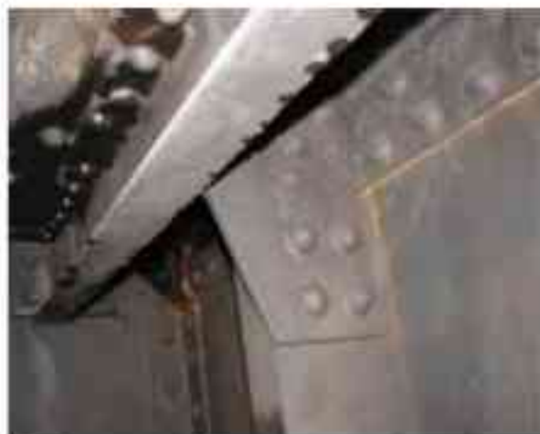
Fig. 5: The corrosion in the interior spaces was predominantly on rivets and crevices.
