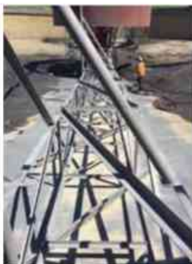
Fig 3: Truss on a rake arm in a final clarifier.
