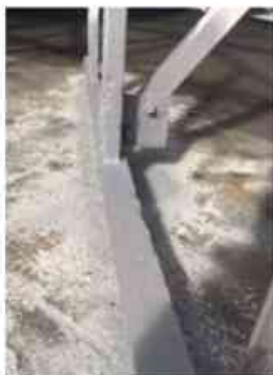
Fig 2: Sweep for a rake arm on a final clarifier.
