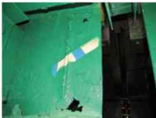
Fig. 3: Paint will need to be removed from this painted-over, masked repair area in order to install the repair.
