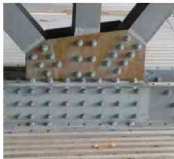
Fig. 11 Flash rusting on a gusset plate resulting from incorrectly applied primer. Photos courtesy of the author.
