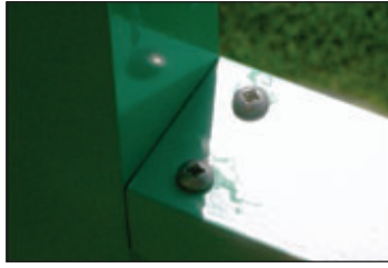
Fig 5: (Case 3) Coating blisters developed where stainless steel screws were used to fasten an aluminum railing to a post.
