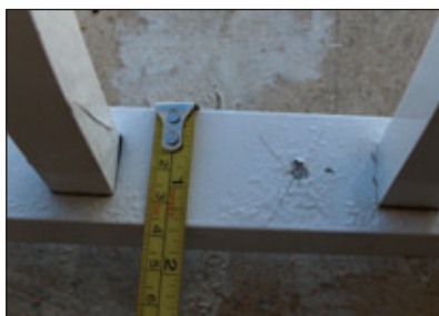
Fig 2: (Case 1) Bottom rail patches of small, irregular blisters between picket penetrations do not appear to be directly linked to filiform corrosion from the edges associated with the penetrations. Not to scale.
