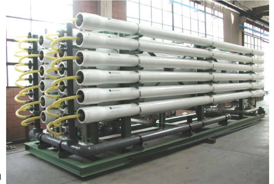
RO rinse waste system
